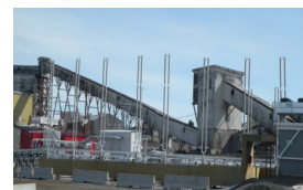
Thermosyphons at Giant Mine (passive heat exchange system that keeps underground arsenic frozen (J.Sandlos))
